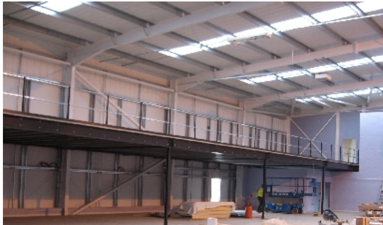
Above a professional installation by our engineers
